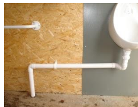
7: Picture of the urinal pipework.
