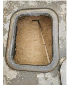
Rake rested inside active vault.
