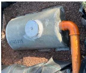
4: The soakaway in position before covering with membrane. Include the pipe connection from the vaults.
