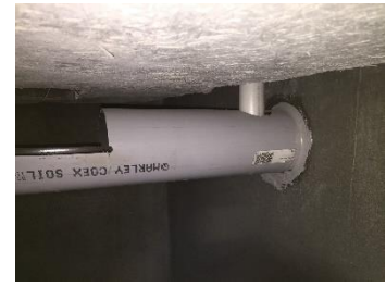
10: Showing that the end of the urinal pipe just enters the urine gutter. It should not go so far in as to block the gutter.
